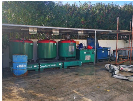
Dangerous Wastes management facilities – Marina
